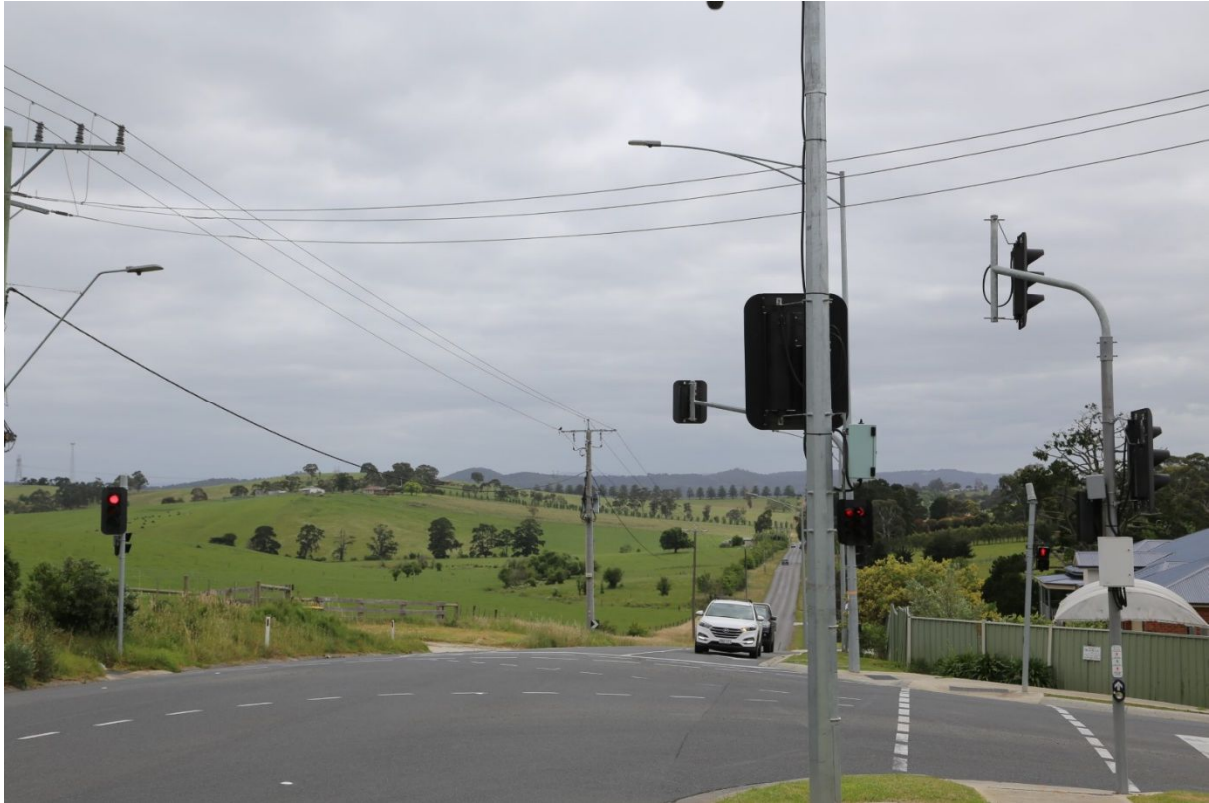
Figure 11 - Existing infrastructure – Existing power infrastructure and lighting poles along Edwards Road. Both Meadow Fair Way and Cherry Hill Way have overhead power infrastructure.
